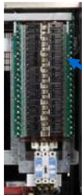
CT Strip mounted to Panelboard
